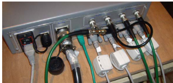
Figure 22 – Ferrite cores set up on the serial cables of the GAPS BOX
