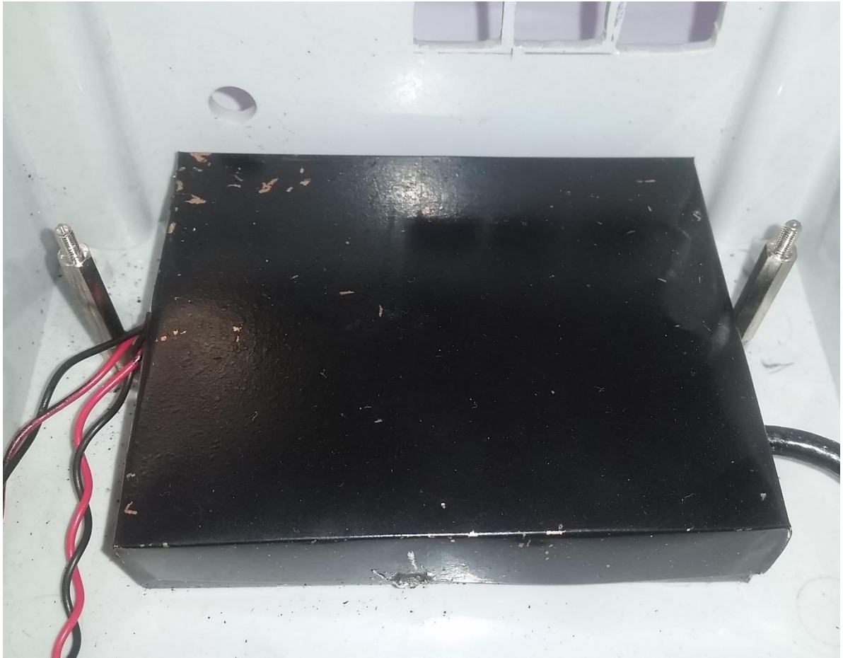
Figure 7: High voltage supply
